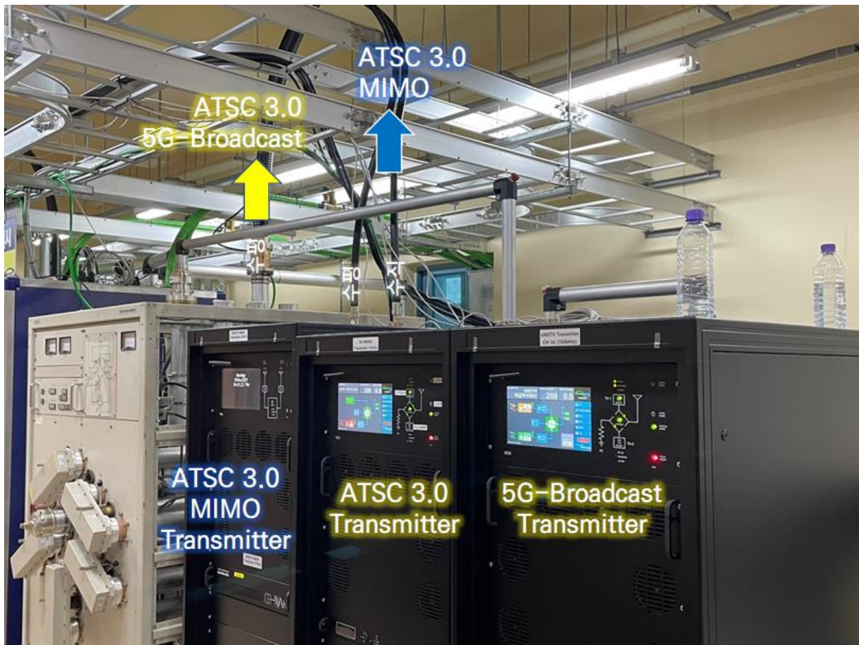
Figure 2.2.5 Experimental transmitters installed at the Bukgamak Experiment Station. ATSC 3.0 MIMO Transmitter capable of transmitting 300W on the left. ATSC 3.0 SISO Transmitter capable of transmitting 900W each in the middle and 5G-Broadcast Transmitter on the right.
