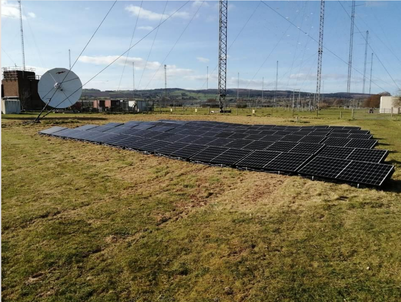
60kWh battery storage (2022)
