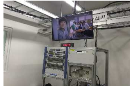
Transmission Site ATSC 3.0 Exciter
