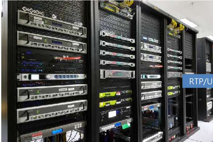
KBS UHD Master Control Room HEVC Encoder ATSC 3.0 IP Multiplexer ATSC 3.0 Broadcast Gateway IEEE 1588v2 PTP Master Clock, etc.
